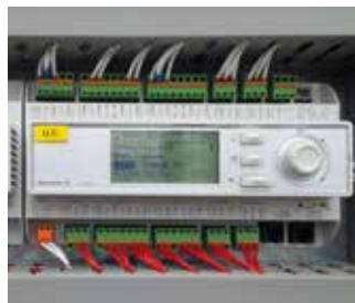
Controller box upgrade
